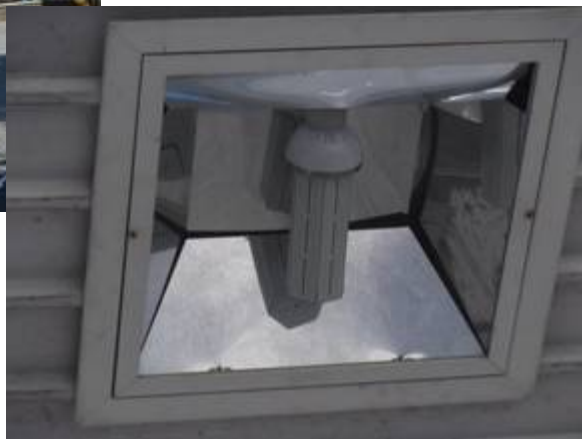
Figure 5.7.2 LED Lighting Units located in Canopy
