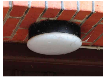
Figure E.10: NonFCO, frosted glass. As installed in this figure, UH: 10-15%, UL:5-10%, ULR: 15%-25%. This type of fixture is often installed vertical on walls, then the ULR increases to 50% with UH: 41%, UL: 9%.
