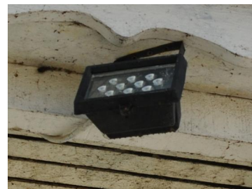
Figure E.1: NonFCO, LED floodlight. Fixture is not FCO and the CCT is to high >3000K.
