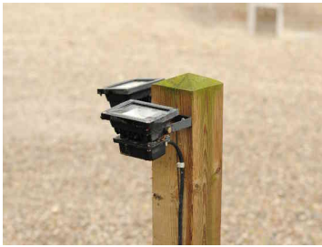
Figure E.28: LED spotlight as uplight below a tree, nonFCO. UH: 100%, ULR: 100%.
