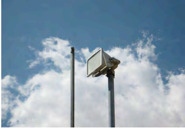
Pole mounted floodlight in Nature Center parking area
