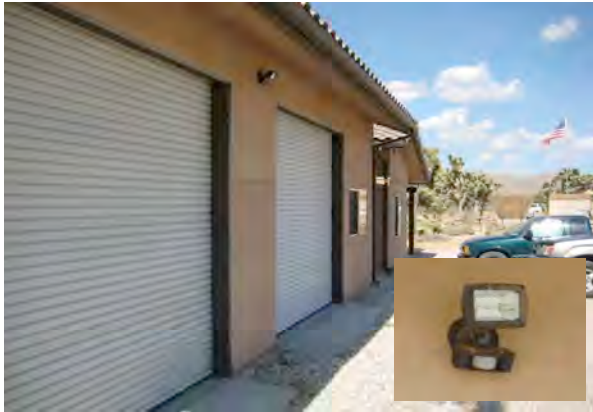
Wall mounted flood light on fire station
