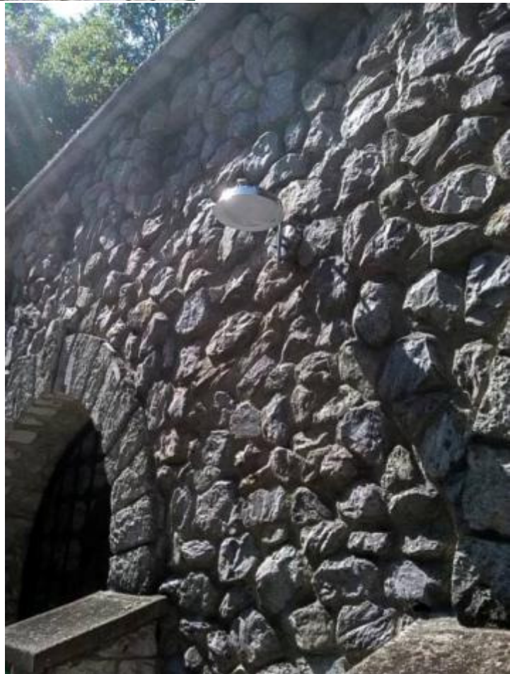
Old and new lighting fixtures, replaced at the entrance of the St. Stephen's Cave (Bükk National Park)
