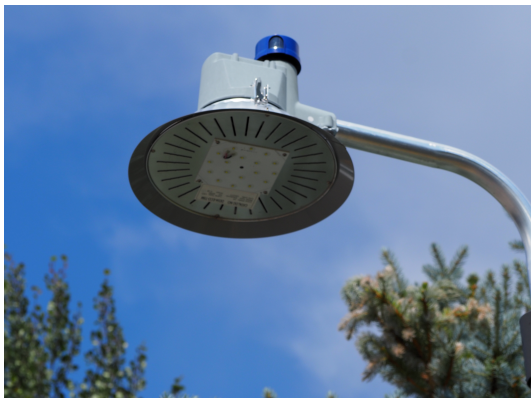
Mountain Village Employee Housing Parking Lot Lights, Stanley.
