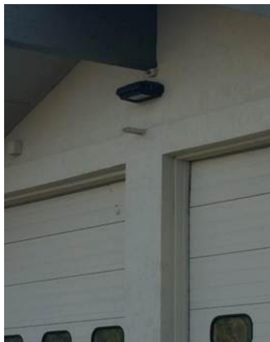
LED Shielded Light Fixture, Sun Valley
