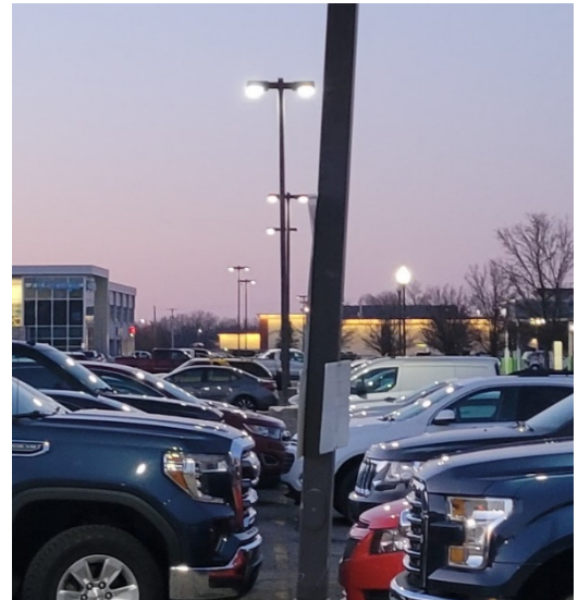
Figure 2-3. Luminaire installation variance.
